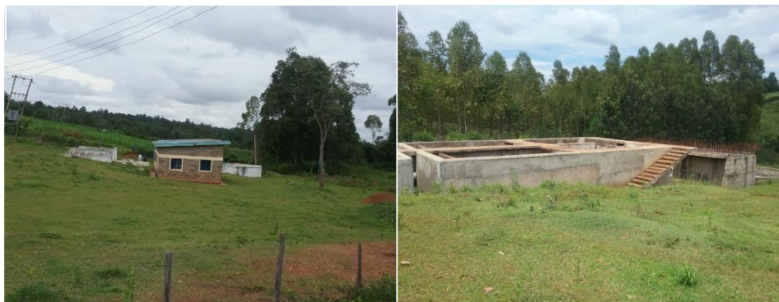
Current and Ongoing Water Treatment Plants
